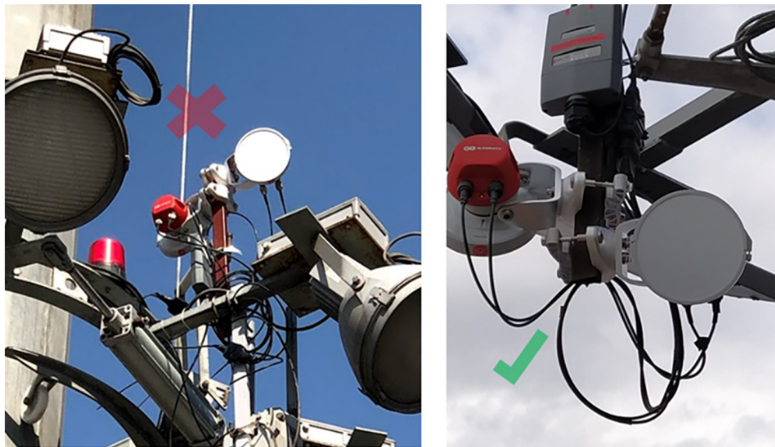
Figure 43: Roll-Out Best Practices: Incorrect and Correct Antenna Installation
