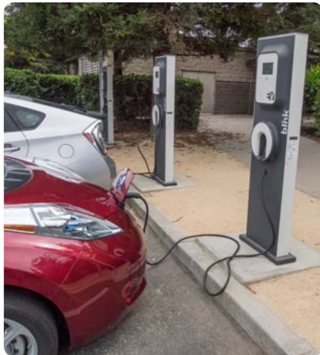
Electric vehicle charging at Cisco (San Jose, California)
